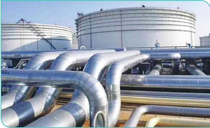
Liquefied Gas Industry
