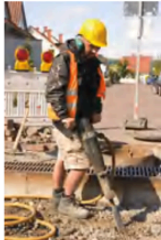
Figure 5 Hearing loss can occur with continuous exposure to loud sounds. Workers in many occupations, such as construction, wear ear protection. The jackhammer this worker is operating has a sound level of 130 dB.
