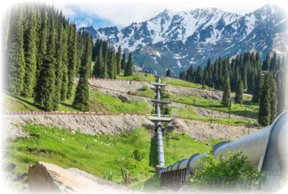
Pipeline on Big Almaty Lake, Tien Shan Mountains, Kazakhstan
